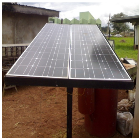
Figure 3 Picture of the Solar PV modules.
